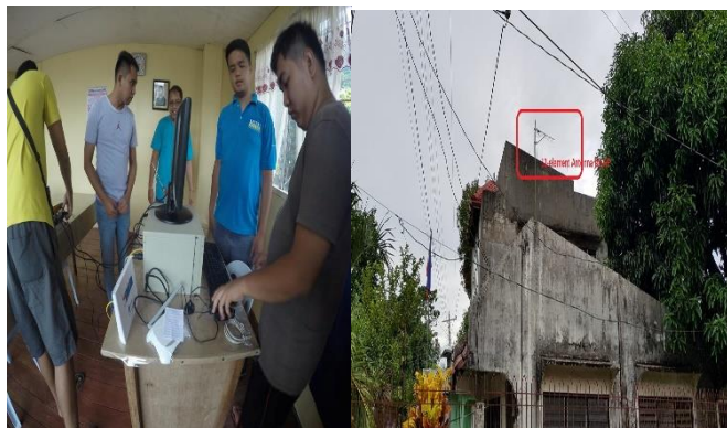
Fig. 7. Configuring the AP inside the Brgy. Hall and placement of the 12-element antenna at the floor just outside where the team has installed the AP.
